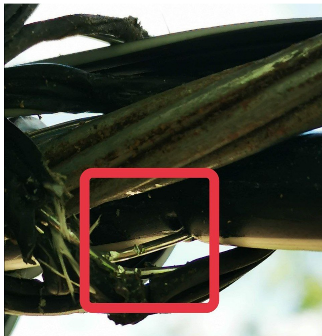
Figure 6. Fiber optic cable partial cut due to pinching of lashing wire
